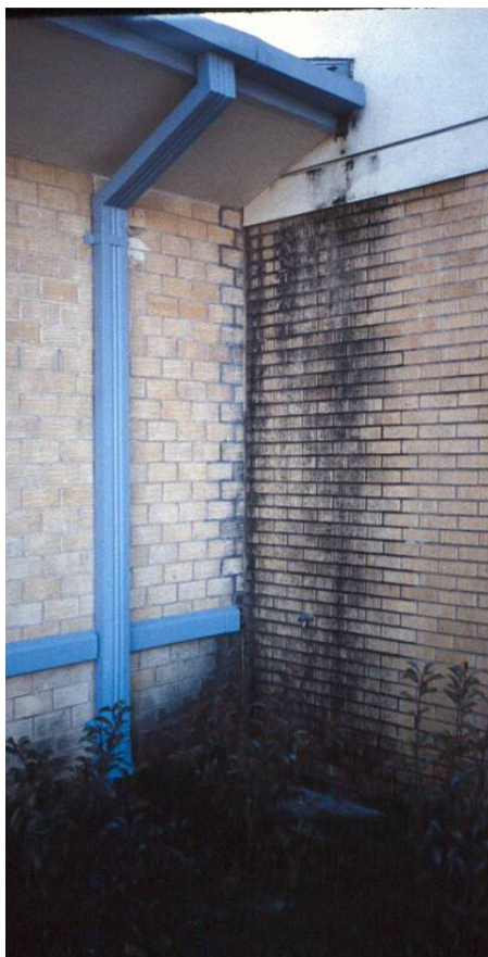
The darkness of the bricks is a good indicator of mold at work.
