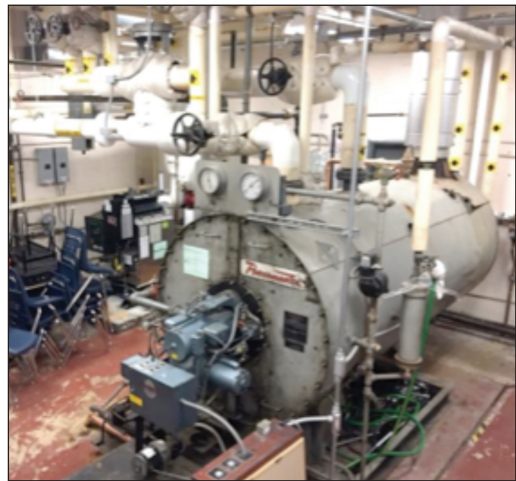
Old boiler used to heat a school.
