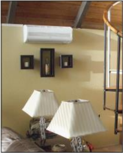
Air handler with blower and heat exchange coil
