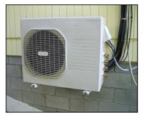
Outdoor unit with compressor and heat exchange coil
