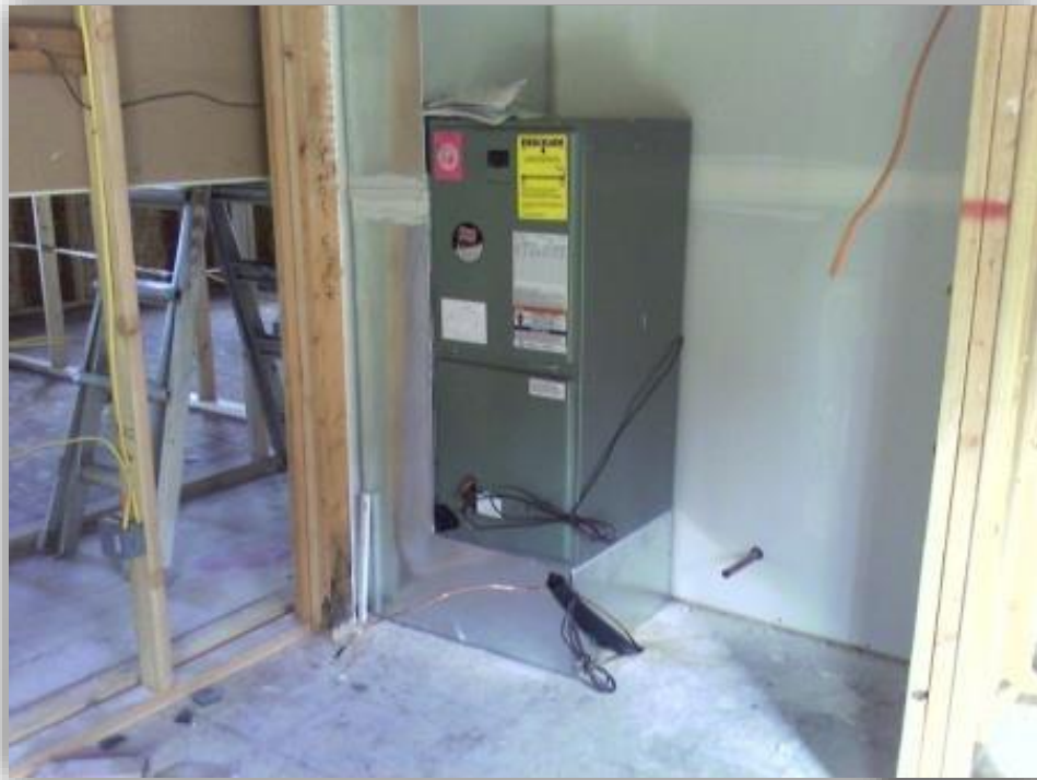
Air handler inside
