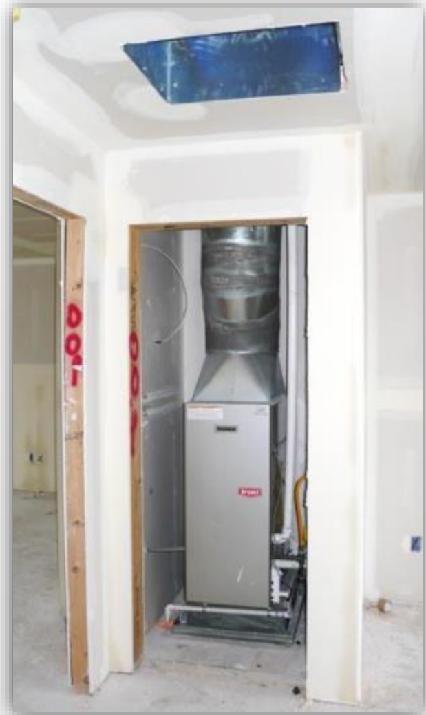
High-efficiency furnace inside the structure
