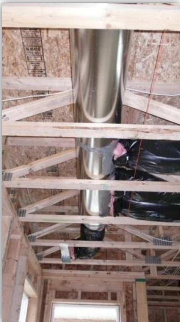
Ducts between floors
